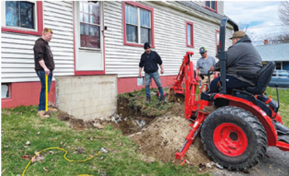
Adrian Russell and Paul Yaskonis of No Job 2 Odd with Greg Niemela, the contractor, stand by while foreman Dakota Drinnon runs the Kubota to finish digging out the space in preparation for a new pressure-treated deck in Keene.
